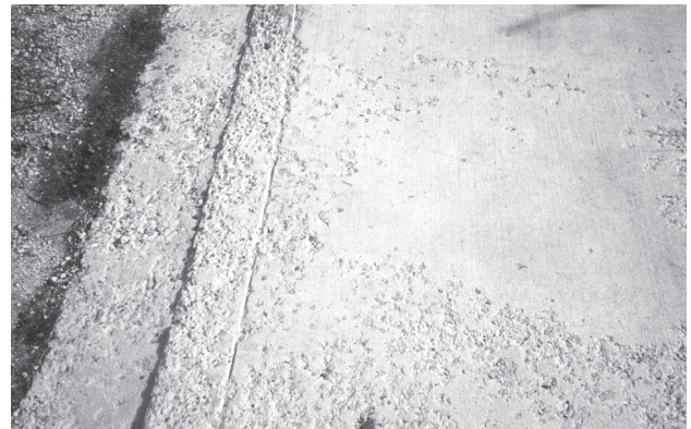
Scaling concrete surface
